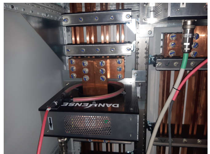
Figure 5: Danisense's DR10000IM sensing head in a Siemens Gamesa wind turbine installation.
